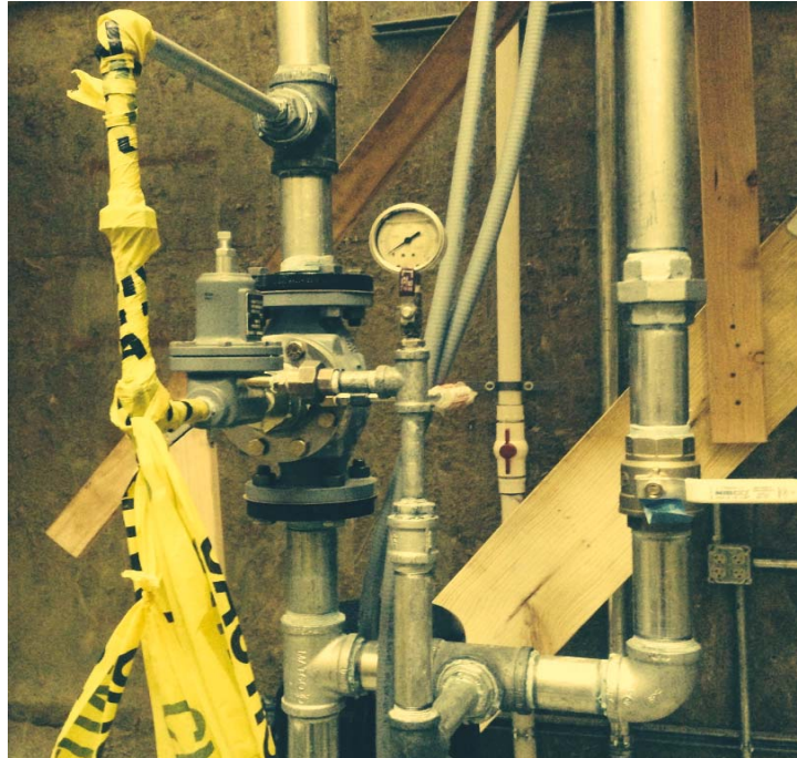
Figure C.2.1 Back-flow pressure valve
