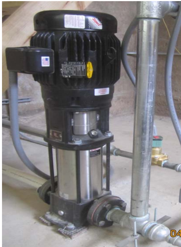
Figure C.2.6 Multi-stage centrifugal pump (10 HP)
