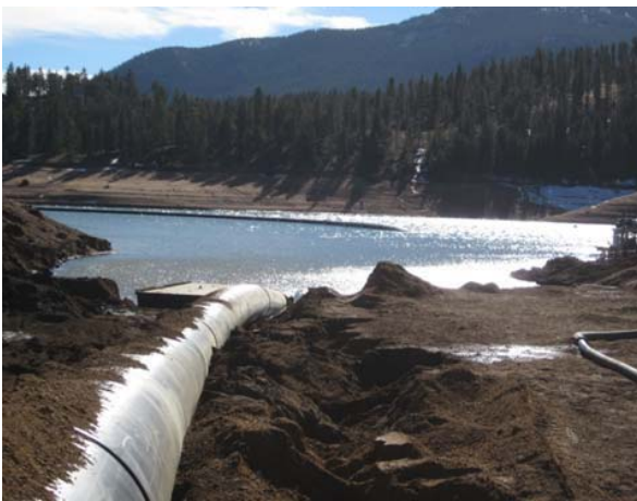
Sinking of pipe on 11-15-2013
