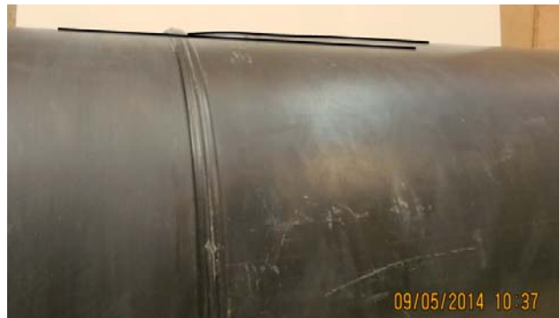
Figure 5.4 Pipe bulge near the middle joint
