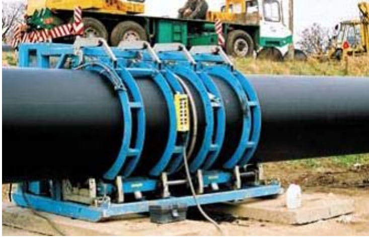
Figure D.3.2 Hot tool butt fusion machine by welding contractor, A.G. Wilson, with (HDPE) PE 100 pipe segments made from Hostalen CRP 100 black
