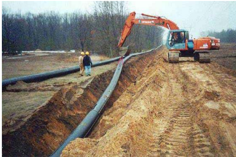
Figure 6.5 Open trench installation of the 20-in. HDPE pipeline that conveys brine solution at 150 psi design pressure
