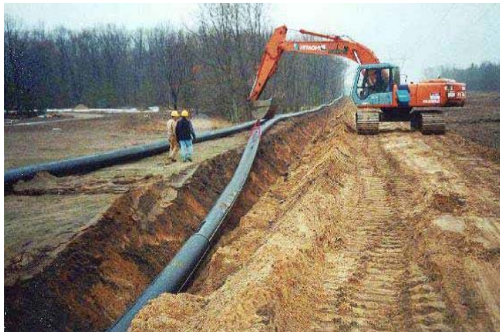
Figure D.4.2 A view of the construction site, where the pipeline was installed open-trench
