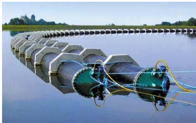
Figure 6.3 A part of the Katrine Lake pipeline spanned a reservoir. Fused pipe segments were sunk down the reservoir using anchoring weights
