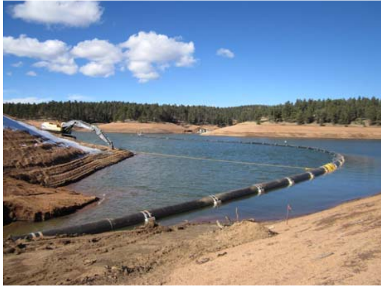
Figure 6.11 Flexibility of HDPE enabled fast construction of the South Catamount reservoir transfer pipeline under a design-build contract
