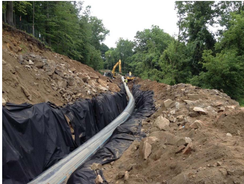
Figure 6.10 Resistance to corrosion and flexibility were the primary reasons for Howard County to select HDPE
