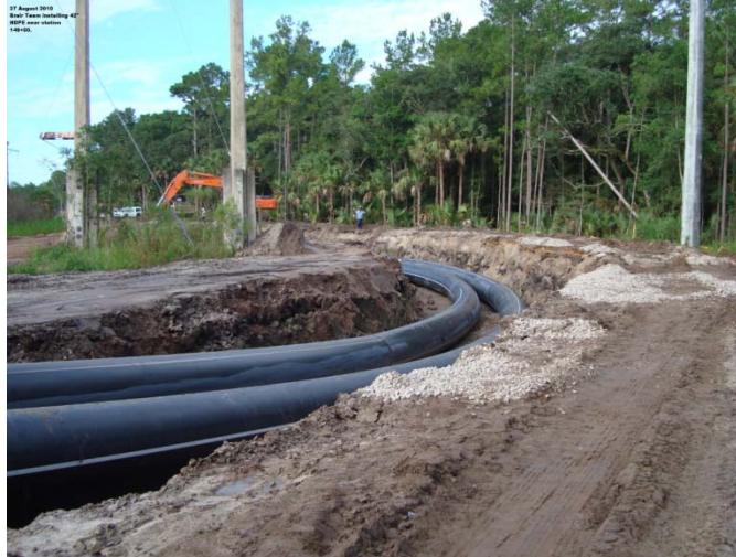
Figure 6.1 A view of a sharp bend that was negotiated with the butt-fused, 42 in., HDPE pipe. Yankee Lake, Seminole County, Florida
