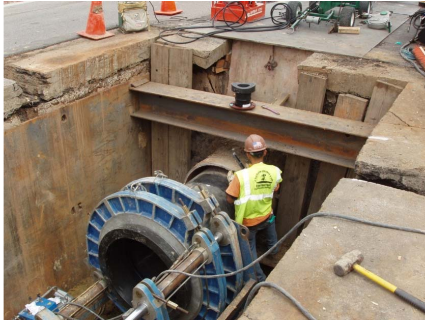
Figure D.1.2 Fusing the joints in the trench imposed a challenge for the construction crew
