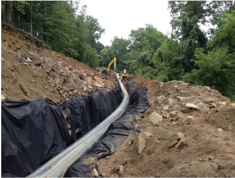
Figure D.10.1 Flexibility was among the reasons for selecting HDPE pipe
