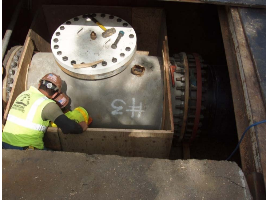
Figure D.1.4 Flanged tee connected to the new HDPE pipe
