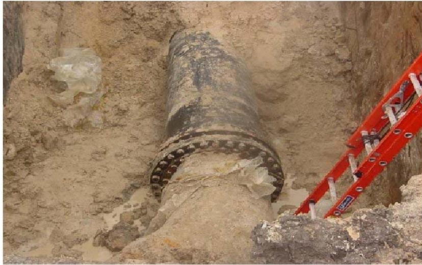
Figure D.5.1 Flanged connection between the 30 in. HDPE and bar wrapped concrete pressure pipe
