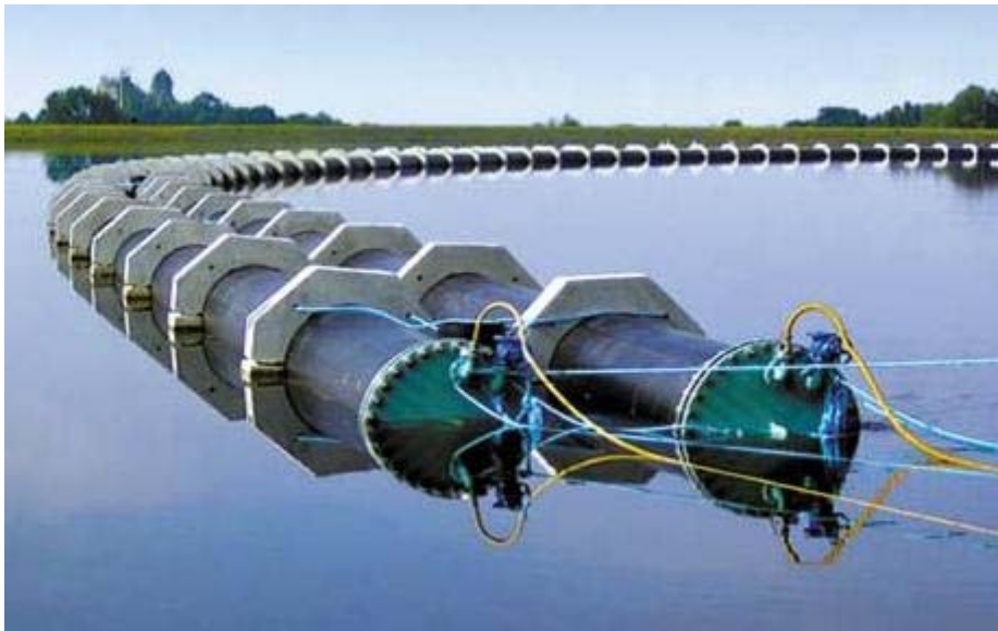
Figure D.3.1 A part of the Katrine Lake pipeline spanned a reservoir and fused pipe segments were sunk down the reservoir using anchoring weigh
